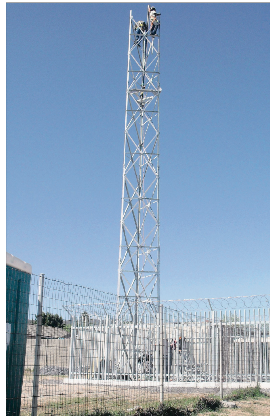
■ The Cell C mast in Steenhoven Street.
